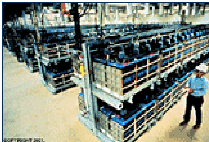
An islanded lead acid battery stack in Alaska
