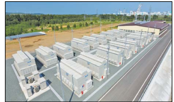
A 34-MW, 245-MWh NaS battery installation.
